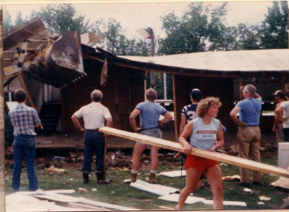
Many in the community turned out for the demolition of the old rink cabin at Dunrobin on Saturday, Sept 10, 1983. One portion was salvaged for future storage use and anything worth saving was sold at an auction on the following Saturday. The Association expresses thanks to Mac Snelgrove for this opportunity.
