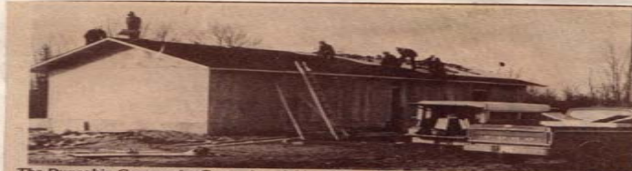
The Dunrobin Community Centre is quickly taking shape by the hard working volunteers on Saturday, Nov. 26th. The centre will hopefully be suitable for skating season scheduled to begin Dec. 19th, 1983.
